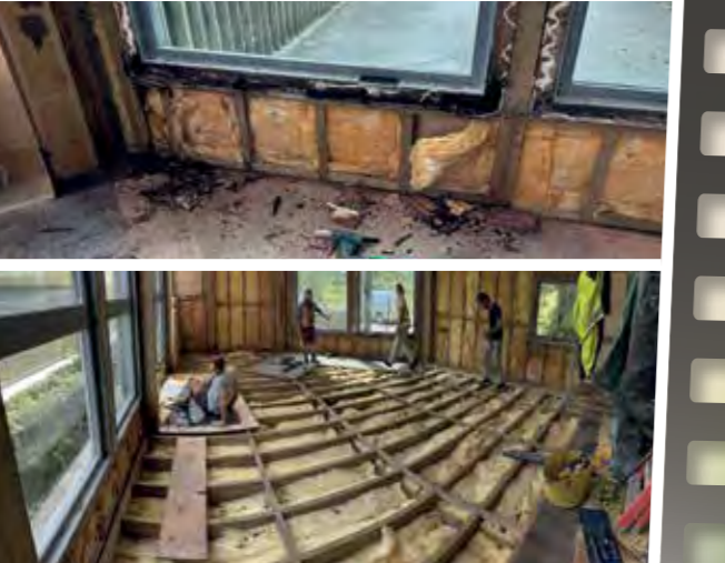
The siamang house needed refurbishment
