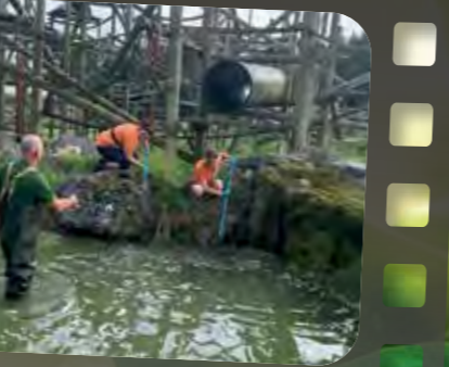
Various ponds (Bart's pond above) needed cleaning out and pumps serviced
